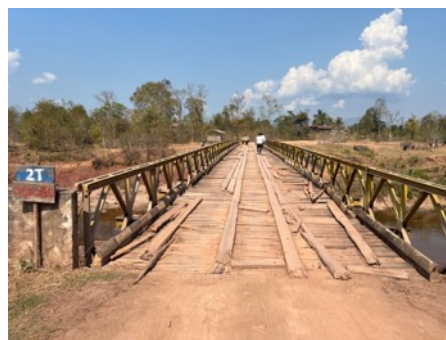
Picture 26 Major steel bridge 60m used to cross the river, carrying capacity only 2 tons.
