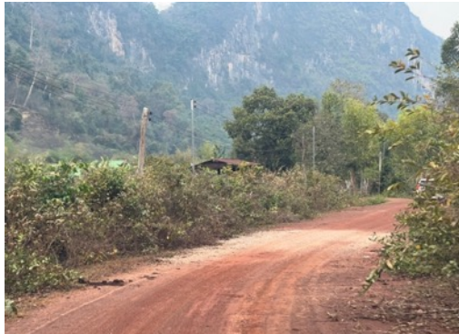
Picture 33 Road 5503 in fair condition however no drainage available.
