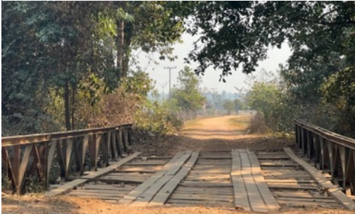
Picture 11 Wood and steel bridge used by community to cross. Carrying capacity
