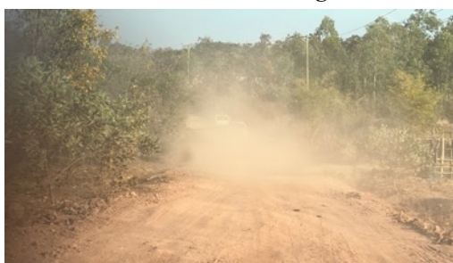
Picture 5 Road 6323 in bad condition with poor drainage
