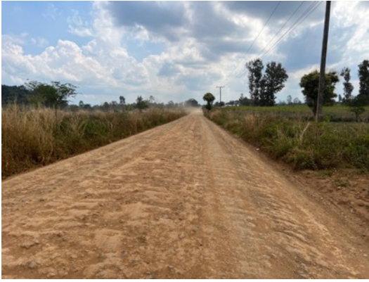
Picture 21: Vegetation on the side of the road blocks drainage. Road 6913.
