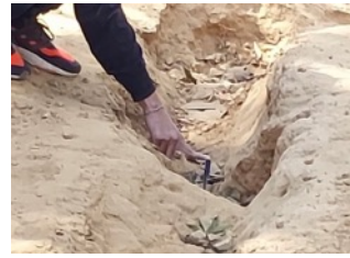
Picture 30 A perspective on the depth of the ruts in the first section of 5675
