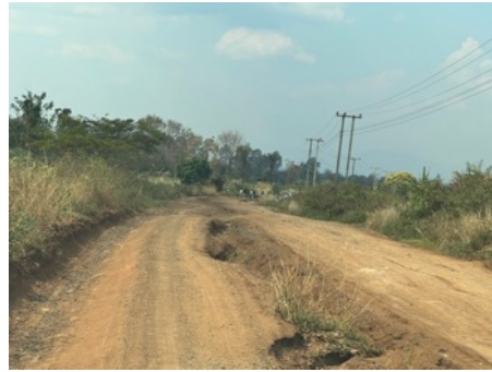
Picture 18 Ruts created by rainfall damage due to poor condition of drainage
