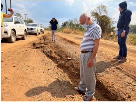
Picture 17 Section of road 6909 damaged by rainfall
