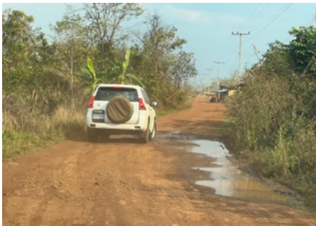
Picture 13 Damage occurring due to local farming practices due to bad condition of drainage
