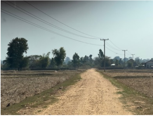
Picture 9 Road 6576 deteriorating due to lack of maintenance, local fauna growing in the road.
