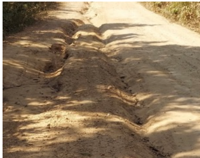
Picture 31 Ruts formed in the first section of 5675 at the mountainous section of the road.
