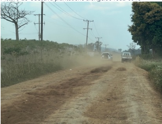
Picture 22 Damage to sections of roads due to heavy rainfall and lack of maintenance. Road 6913
