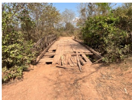
Picture 27 Timber bridge unusable by 4W transport due to heavy damage.
