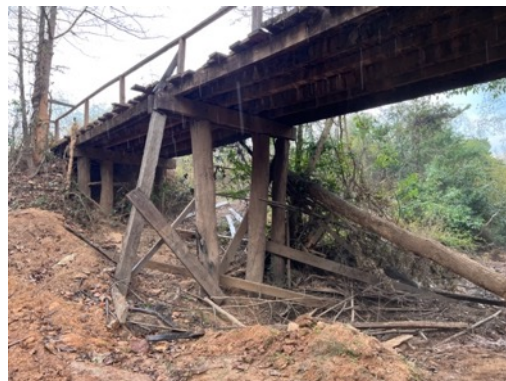
Picture 38 The deteriorating condition of timber bridges in road 5683.
